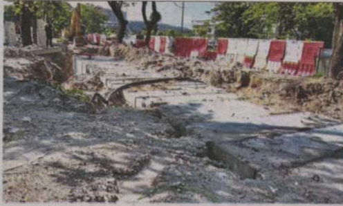
The flood mitigation project site at Jalan Kenari 1, Puchong Jaya.
